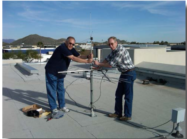
DVPA Directors George Zukauckas and Chuck Crinnian are shown installing a VHF antenna on the roof of the Deer Valley Terminal Building as part of the Sounds of DVT project.
